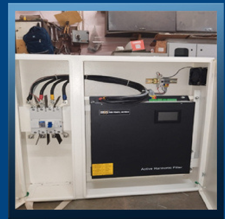
Solar ACDB Harmonics Filter
